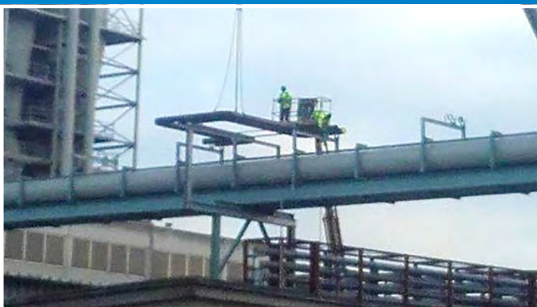
Sonae Arauco, Beeskow plant Thermal oil pipeline Pump room - installation of DN 200 pipeline 2020
